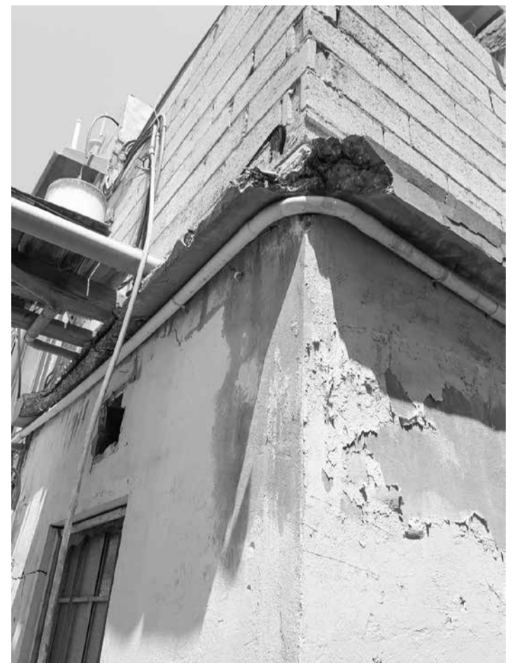
The house can collapse anytime.
